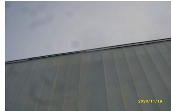
Missing trim to gym cladding
