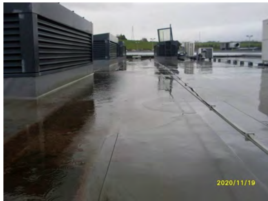
General view—water laying on roof
