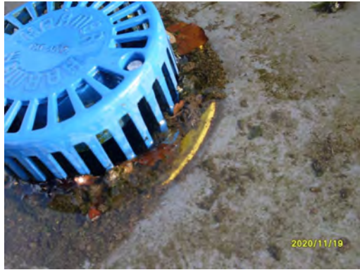
Slow draining roof gully
