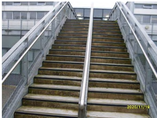
Stair risers requiring cleaning
