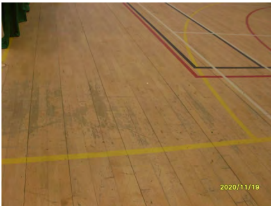
Wear to gym floor
