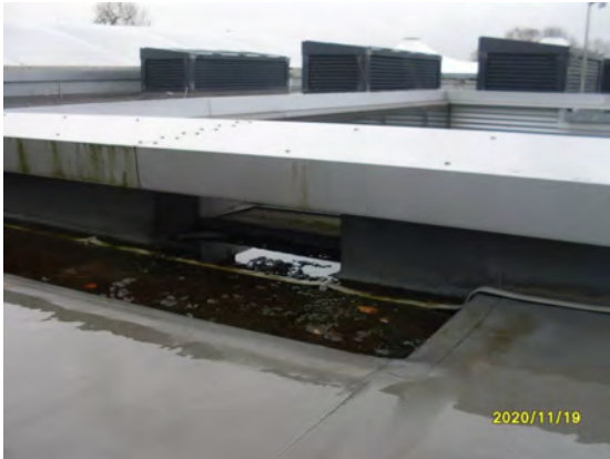
Blocked outlet and ponding
