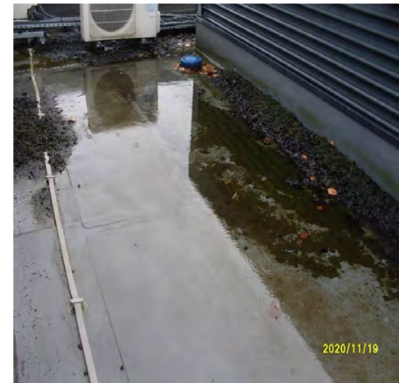
Ponding water and detritus
