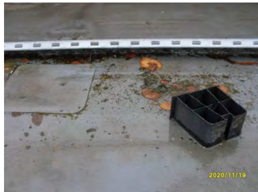
Displaced cable tray support
