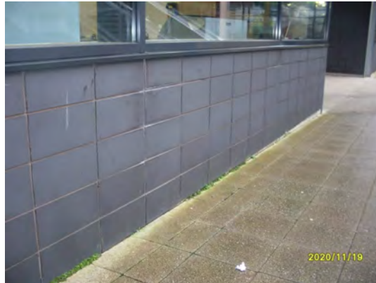
Water run-off and staining to blockwork
